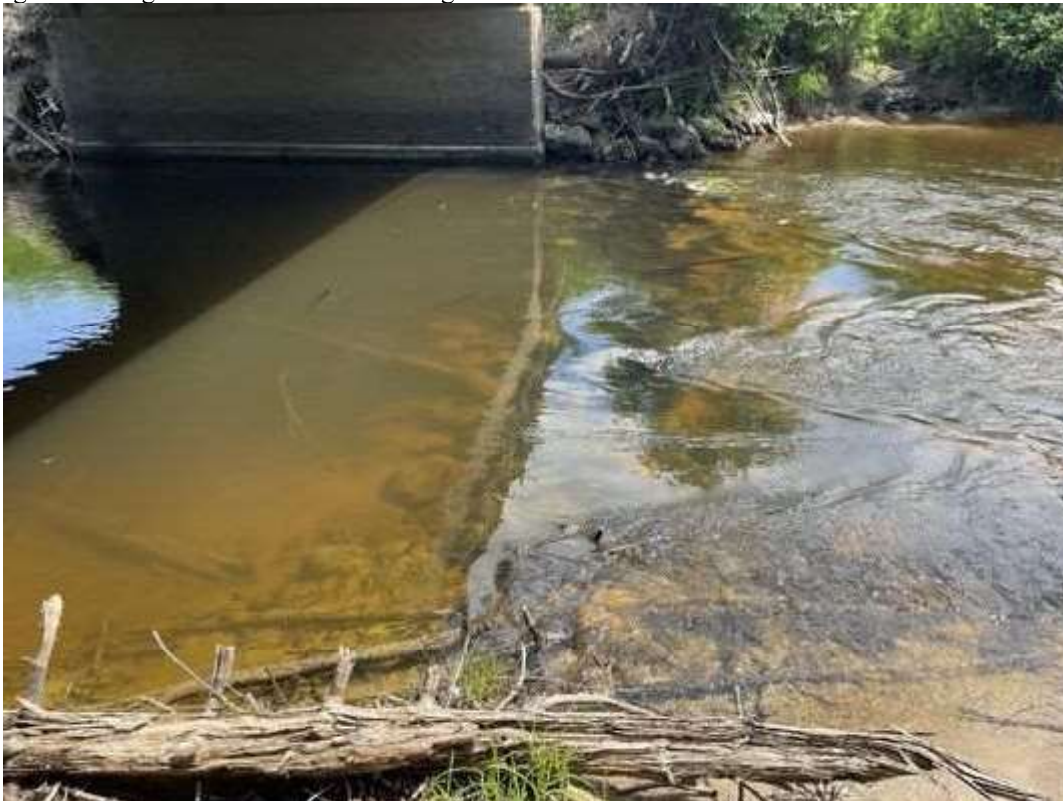
Photo 1: Light damming at the northwest stream edges.
