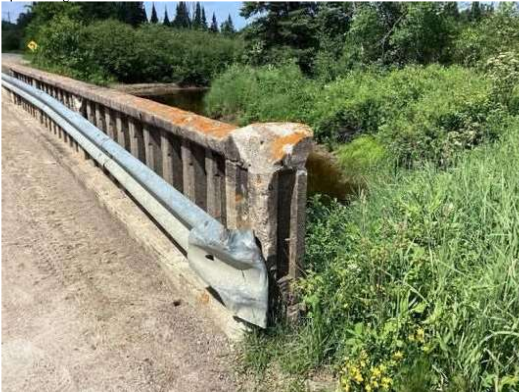
Photo 1: Impact damage at southeast rail.
