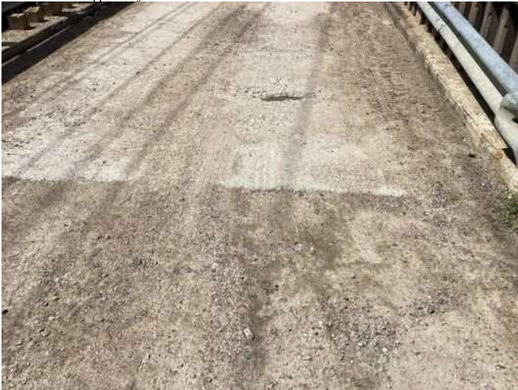
Photo 1: Wheel ruts at the approach joint.
