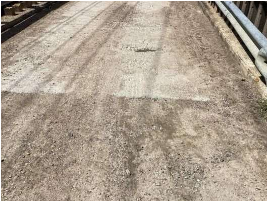
Photo 1: Severe wear and abrasion in the north deck section.
