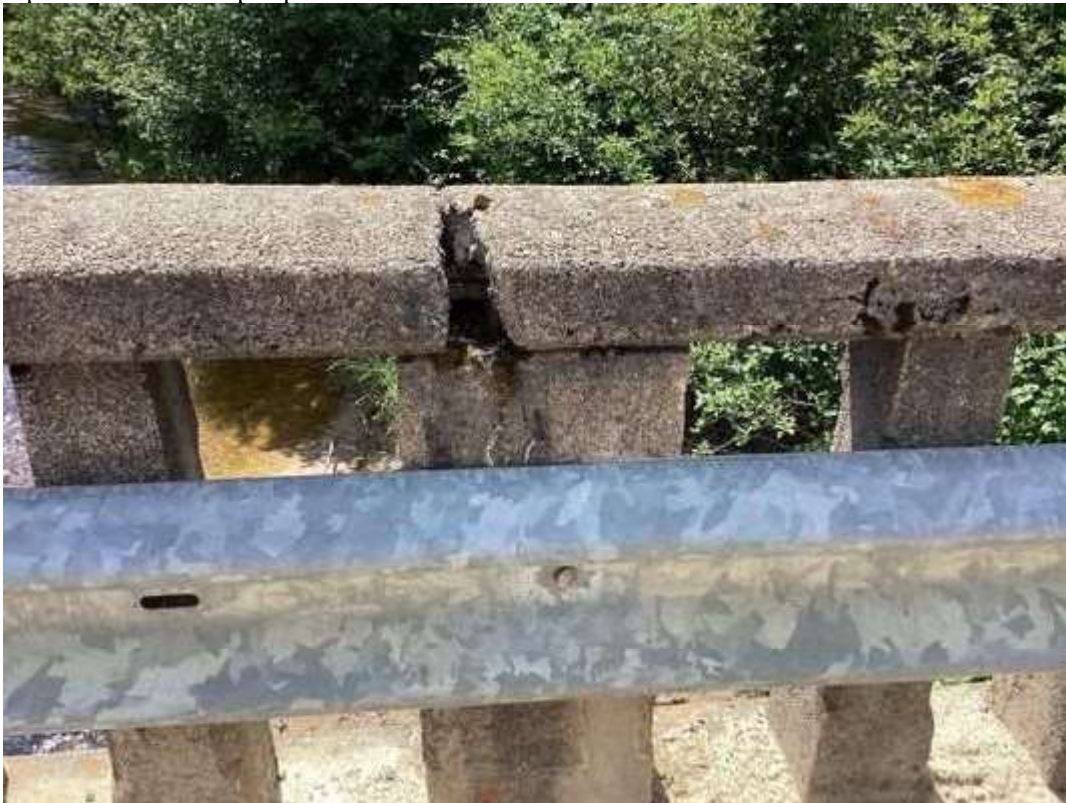
Photo 2: Exposed rebar at west parapet.
