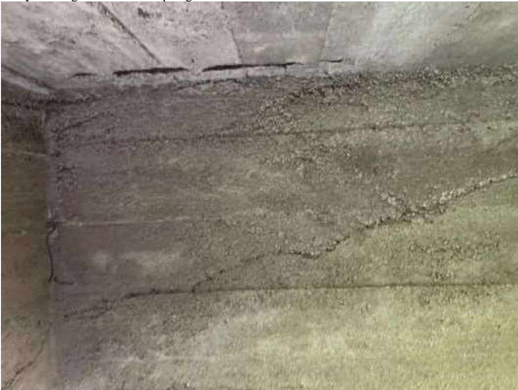
Photo 2: Honeycombing at north end diaphragms.
