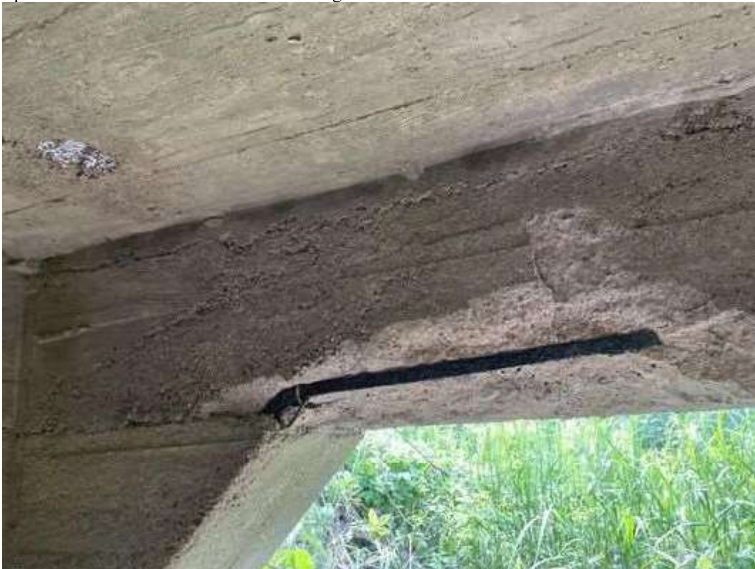
Photo 1: Exposed rebar and severe corrosion at south girder.
