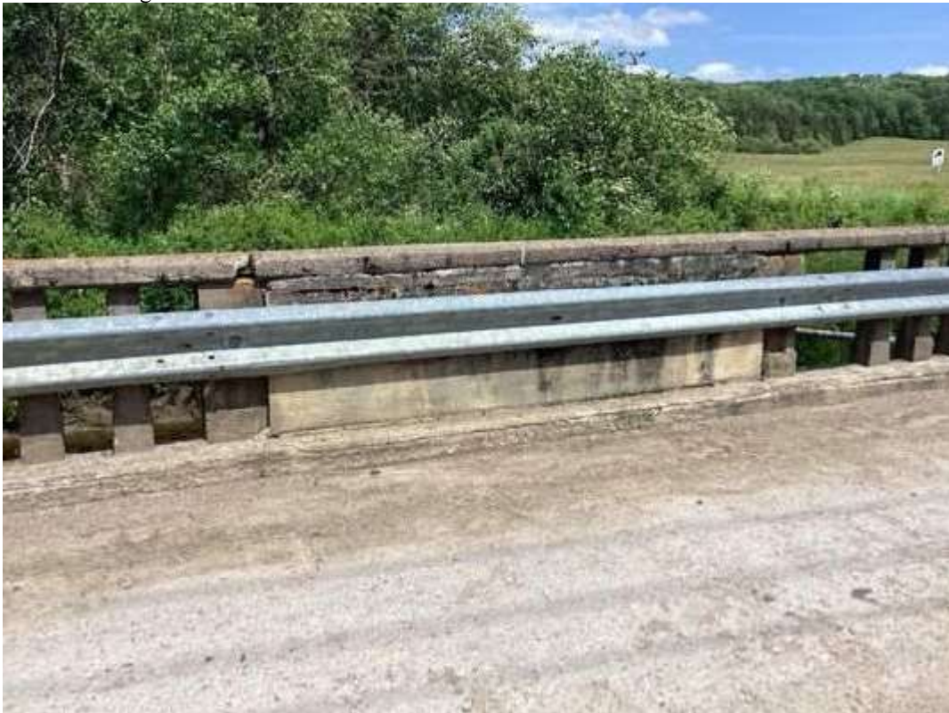
Photo 2: Abrasion throughout north curb section.
