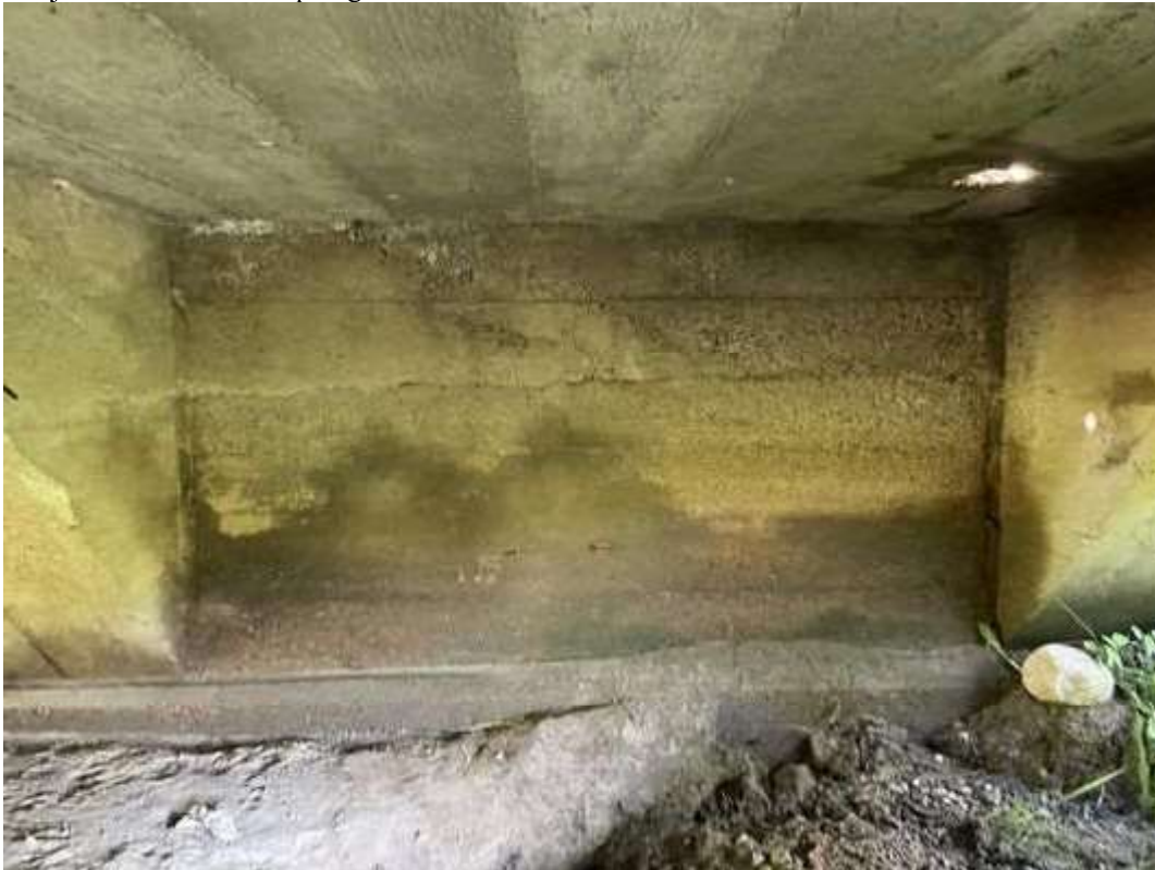
Photo 1: Cold joint at south end diaphragms.
