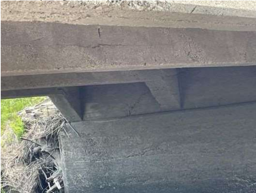
Photo 1: Cracks and honeycombing at southeast diaphragm.
