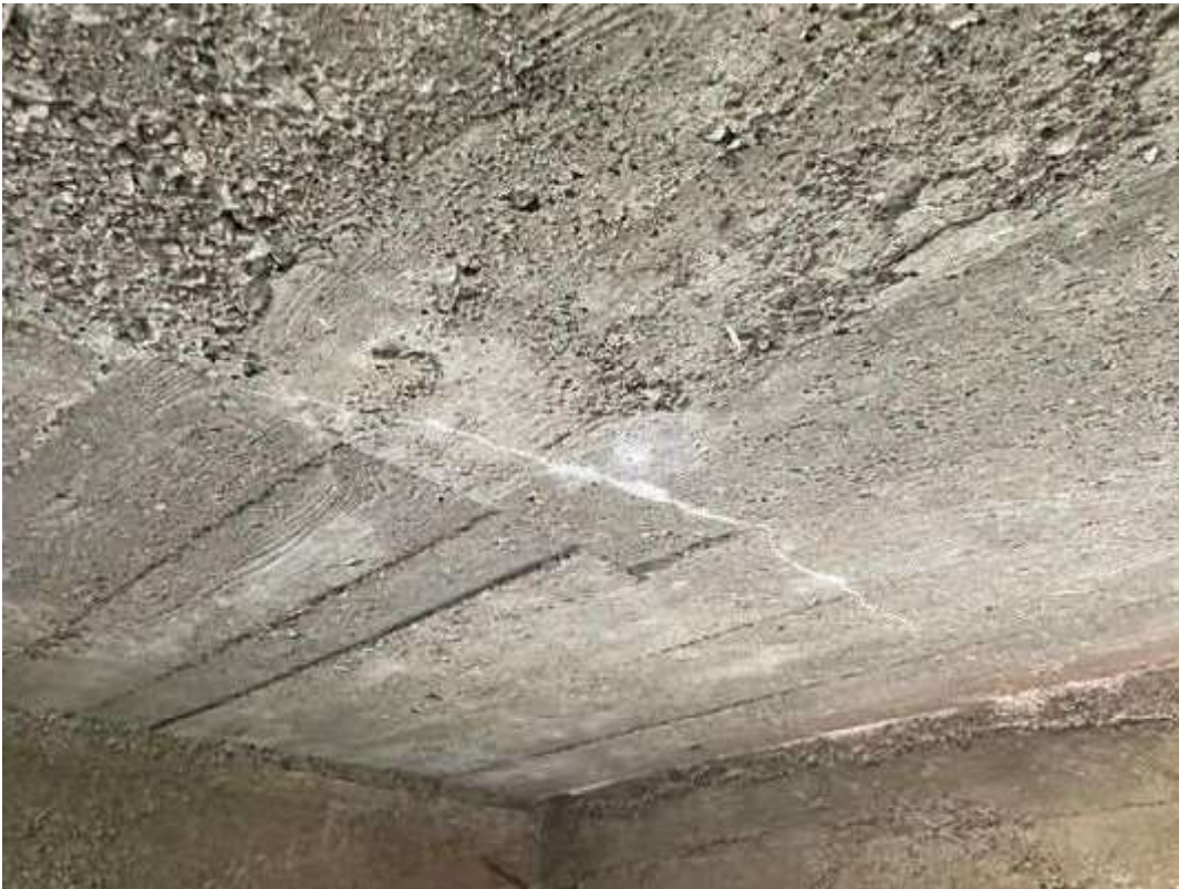
Photo 2: Efflorescence at the southwest soffit.
